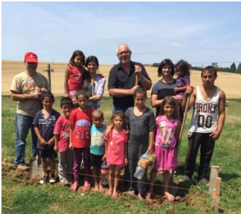
Florin Aslovici, Ari Robotin, Lars Gustavsson and Valentina Ferche together with children and young people in the Roma community when the first ground-breaking dig was made for the construction of a hygiene centre.
